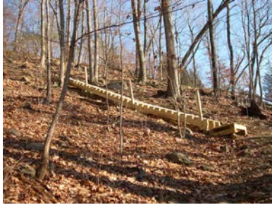
Y2 – Trail erosion at staircase
